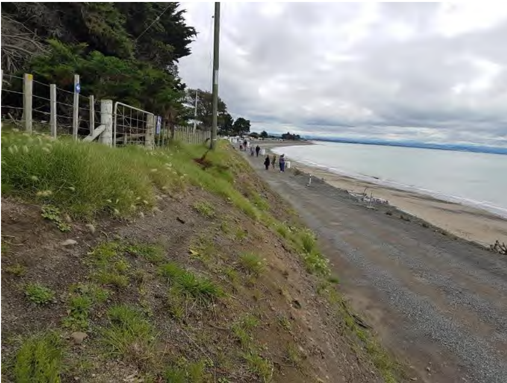
Figure 10 Extent of road cut rendering the archaeological risk in some areas of the revetment low to zero, although risks associated with the road re-alignment remain high (Source: G. Carter).
