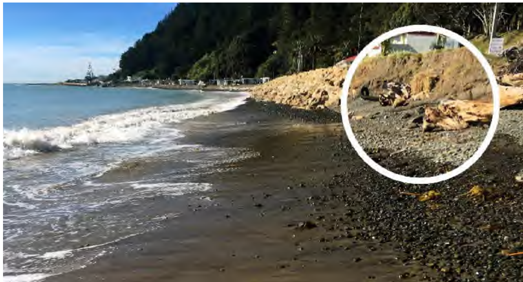
Figure 10: Habitat Adjacent to Existing Revetment (Inset Showing Example Pebble/Gravel Field Habitat Affected by Downdrift Erosion and Likely to Occur Downdrift of the Proposed Revetment).
