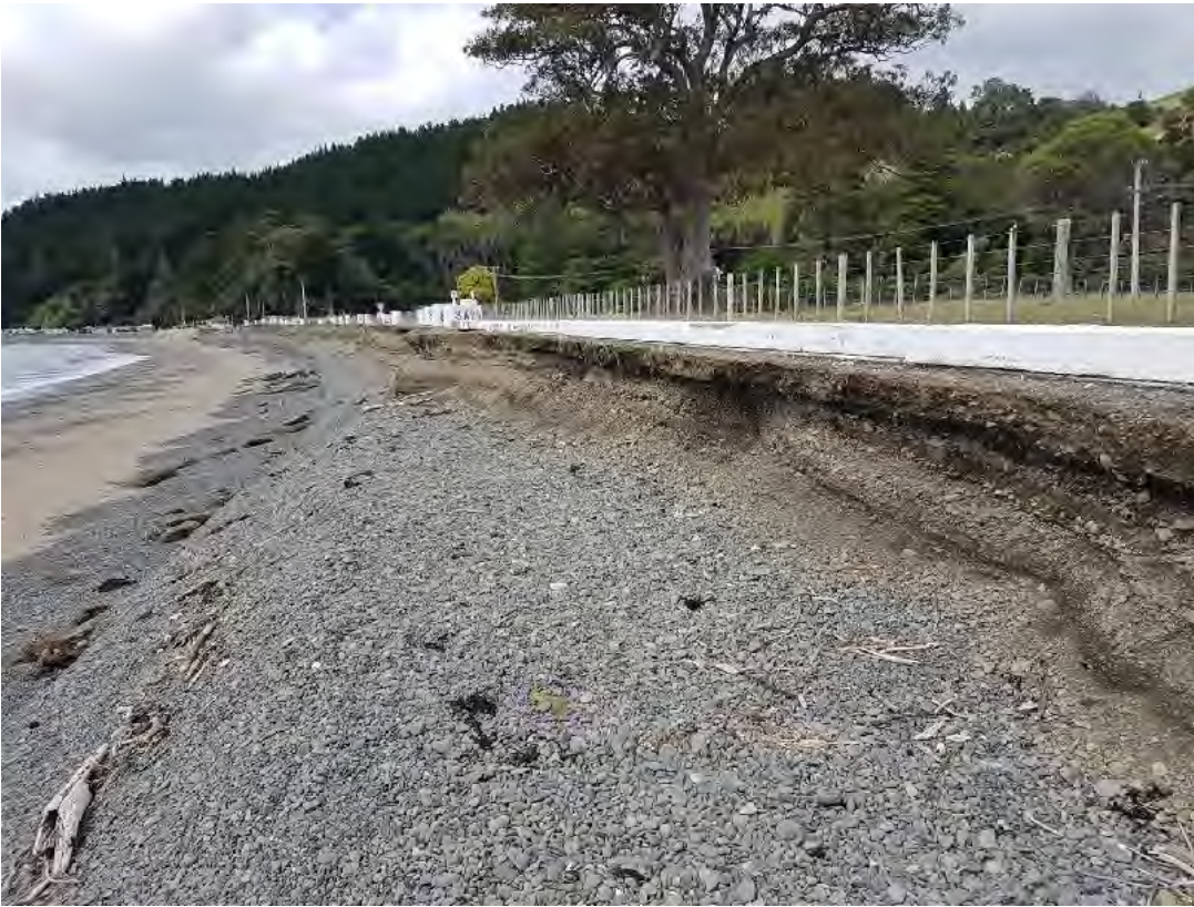
Figure 11 Road and proposed revetment wall level in relation to the existing ground surface in the vicinity of the café end of works (Source: G. Carter).
