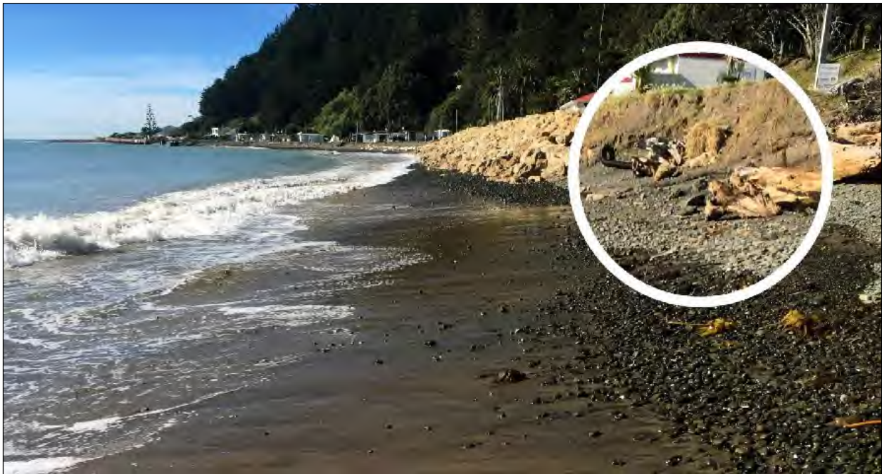
FIGURE 6: HABITAT ADJACENT TO EXISTING REVETMENT; INSET SHOWING EXAMPLE PEBBLE/GRAVEL FIELD HABITAT AFFECTED BY DOWNDRIFT EROSION AND LIKELY TO OCCUR DOWNDRIFT OF A PROPOSED REVETMENT.
