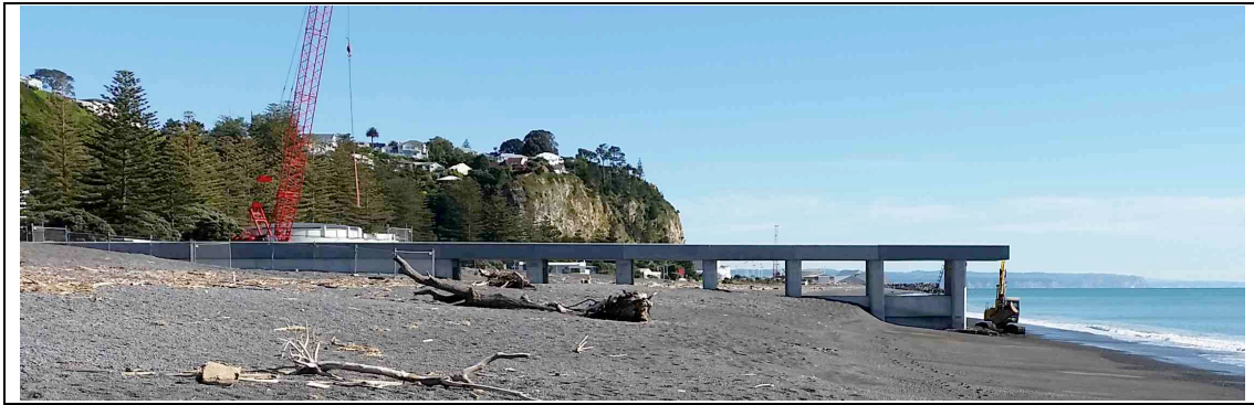
Figure 2.15 Viewing platform under construction on Marine Parade, November 2015 (photo by Zorn Surveying Ltd).
