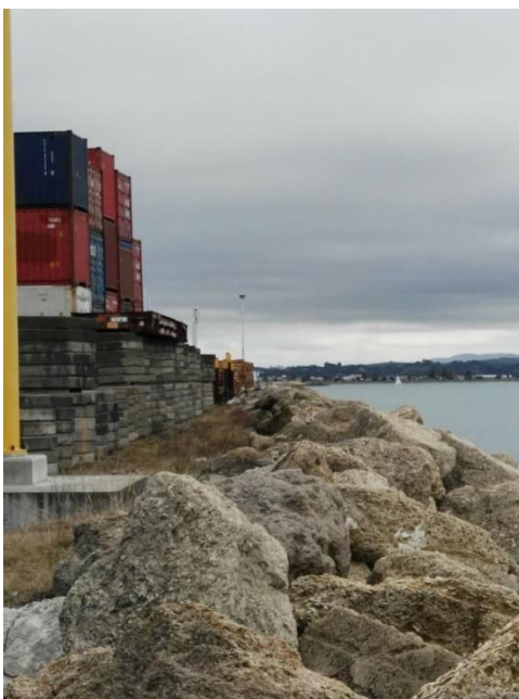
Plate 1: Revetment wall to be affected, showing limestone boulders which will be removed as part of wharf construction.
