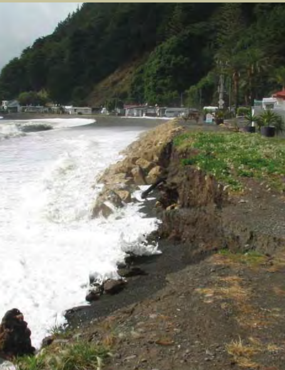
Erosion on the north side of the seawall (photo looking south)
