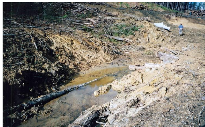
Example of disturbance of the stream bed with debris and sediment from uncontrolled earthworking & harvesting operations
