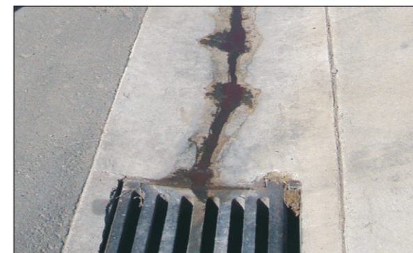
Stains on concrete are evidence of stormwater pollution occurring.
