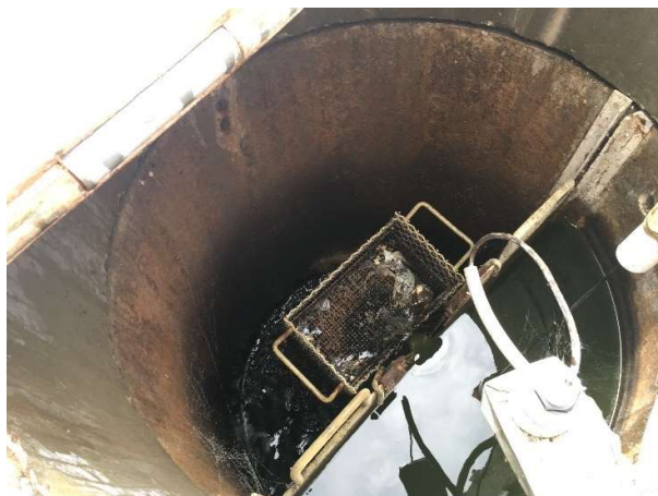
Figure 3 - Effluent discharge chamber and flow meter Transducer
