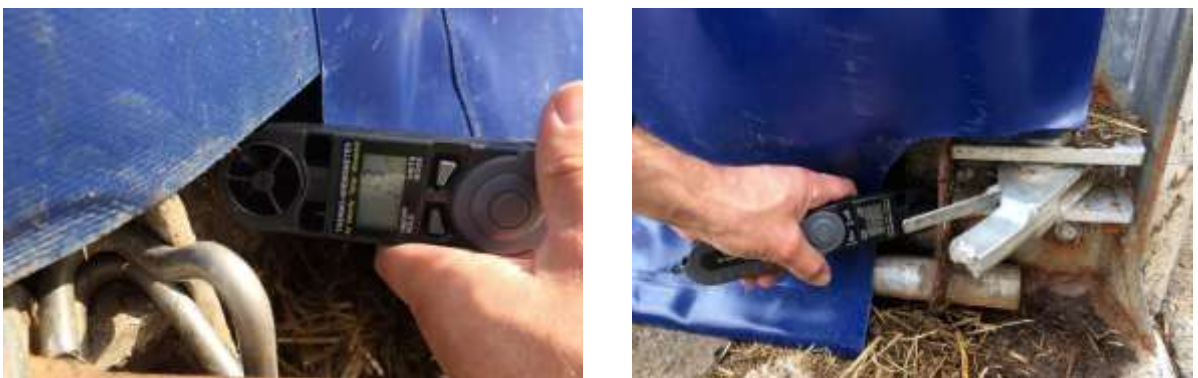
Air velocity tests at openings around doors when doors are closed – all tested air velocities exceeded 0.5m/s – of air being sucked *into* the bunkers.
