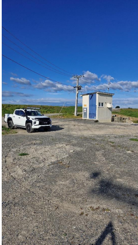
Photograph 1: General view of pumpstation in the carpark, facing southwest.
