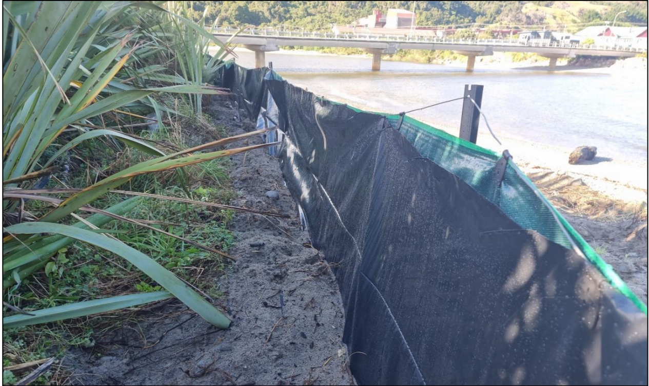
Figure 4. Lizard exclusion fence, showing buried toe of polythene and polythene extending up the silt fence (File Photo).
