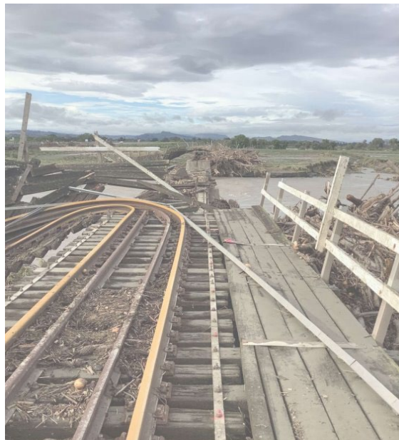
Figure 4: Bridge 217 PNGL damage post Cyclone Gabrielle (Source: TREC)
