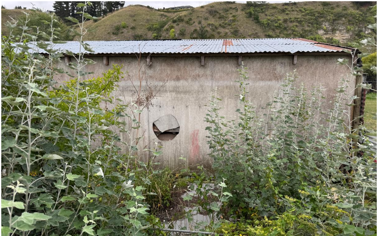
Figure Appendix B.16: Suspected asbestos board on shed at rear of 157 Taihape Road on 28 February 2025. The suspected asbestos was observed to be in poor condition.
