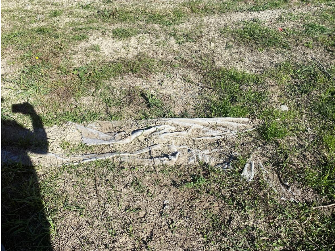
Photograph Appendix B.11: Exposed geofabric present in the paddock next to 203 Taihape Road on 8 May 2024.
