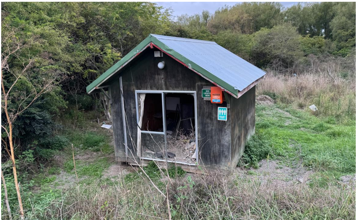
Photograph Appendix B.24: Flood damaged shed at 209 Taihape Road on 28 February 2025.
