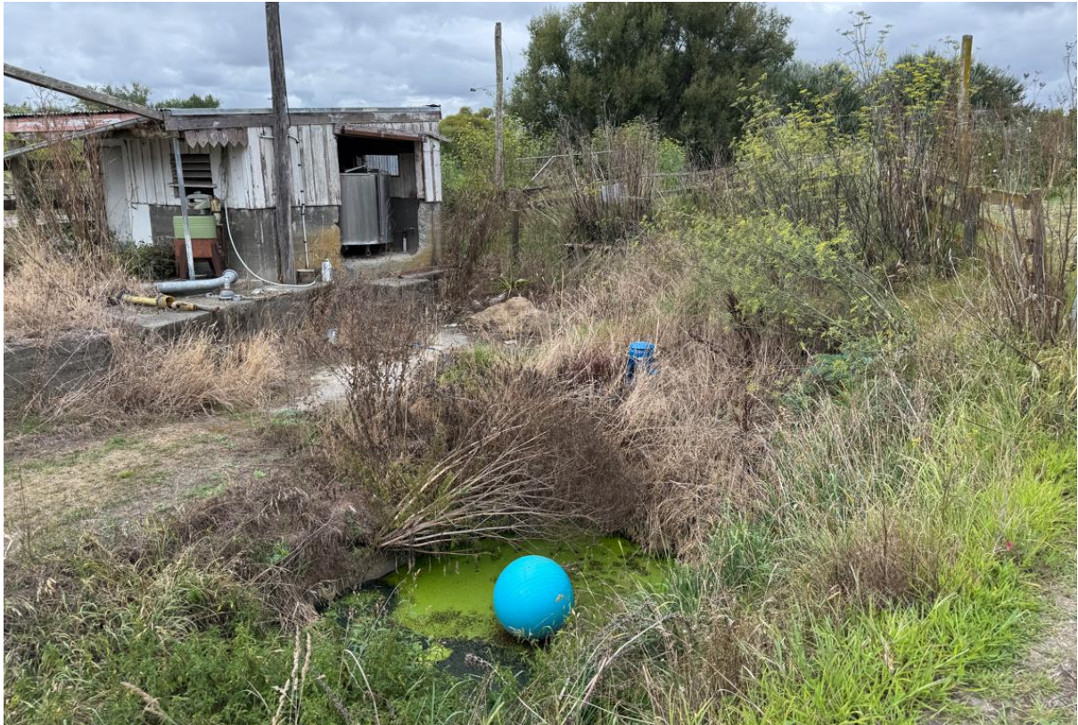
Photograph Appendix B.19: Suspected asbestos cladding on shed at the rear of 131 Taihape Road on 28 February 2025. The suspected asbestos was observed to be in poor condition. An assumed water pump and surface water body is present near the gate in the left of the photograph.
