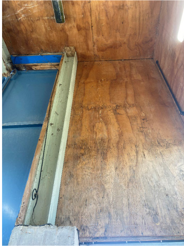
Photograph 9: Interior of the taller pump station building, showing remaining wetness on the ceiling from the flood.
