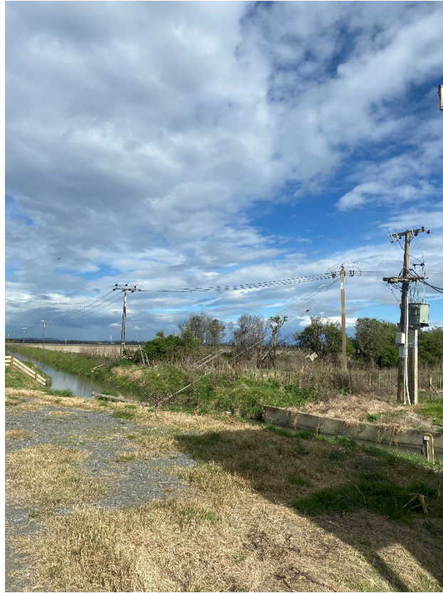
Photograph 5: View of the overhead power lines running south-west along the edge of the main drain channel, supplying power to the pump station.
