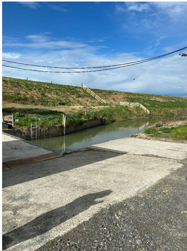
Photograph 6: Overhead cables connected to the taller pump station building.
