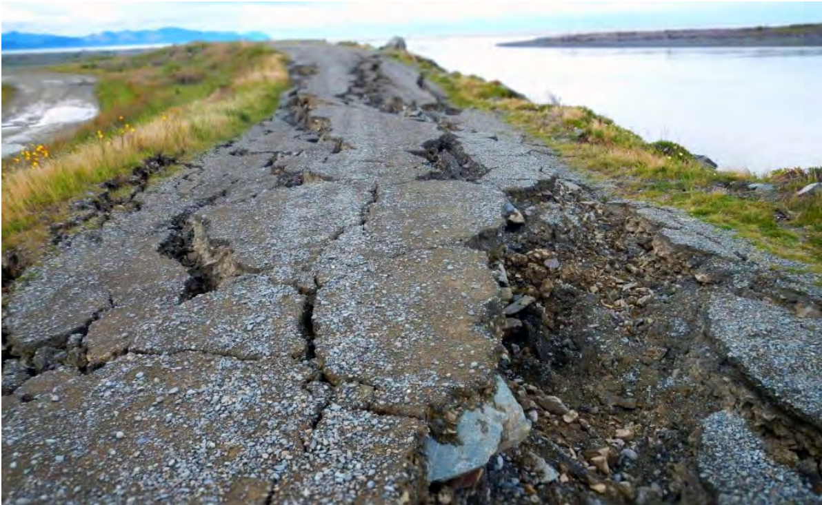
Figure 5.1: A photo showing lateral spreading along a flood protection system 20 .
