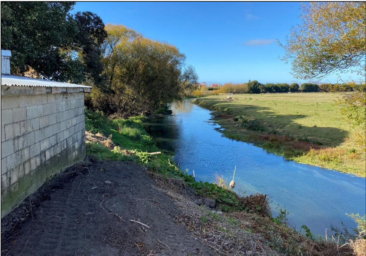
Photograph Appendix B.2: Rear of Pakowhai Hall building beside Tūtaekurī Waimate Stream. Broken fibre cement fascia along rear of building and three fragments visible on ground surface.
