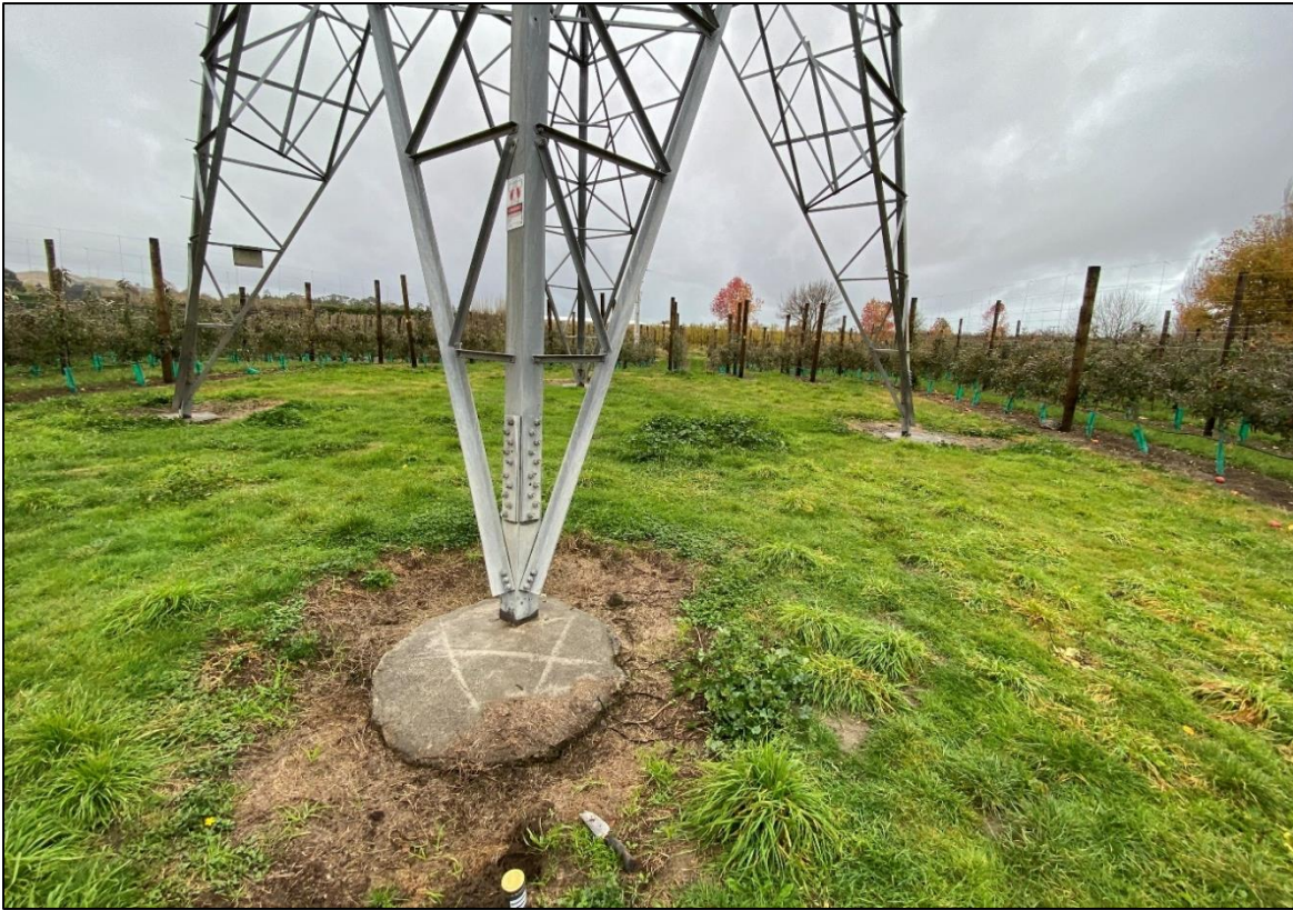
Photograph Appendix B.17: Pylon within orchard at 70 Franklin Road. Sample location SS19.
