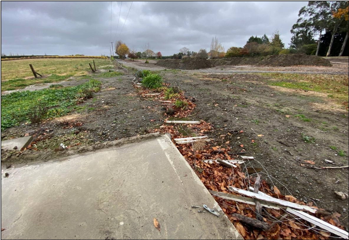
Photograph Appendix B.21: Stockpiles of topsoil in area of earthworks occurring on golf course property, adjacent to 1153 Links Road.
