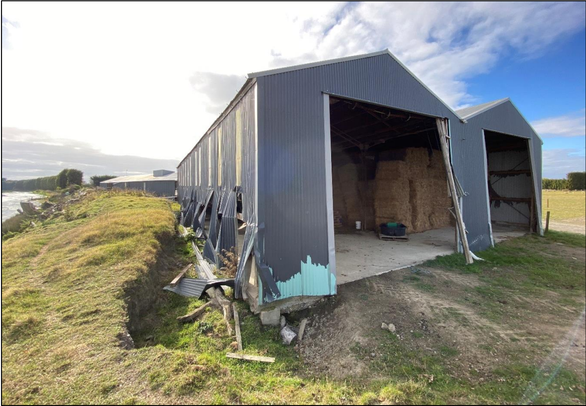
Photograph Appendix B.5: Damaged farm shed at 1854 Pakowhai Road.
