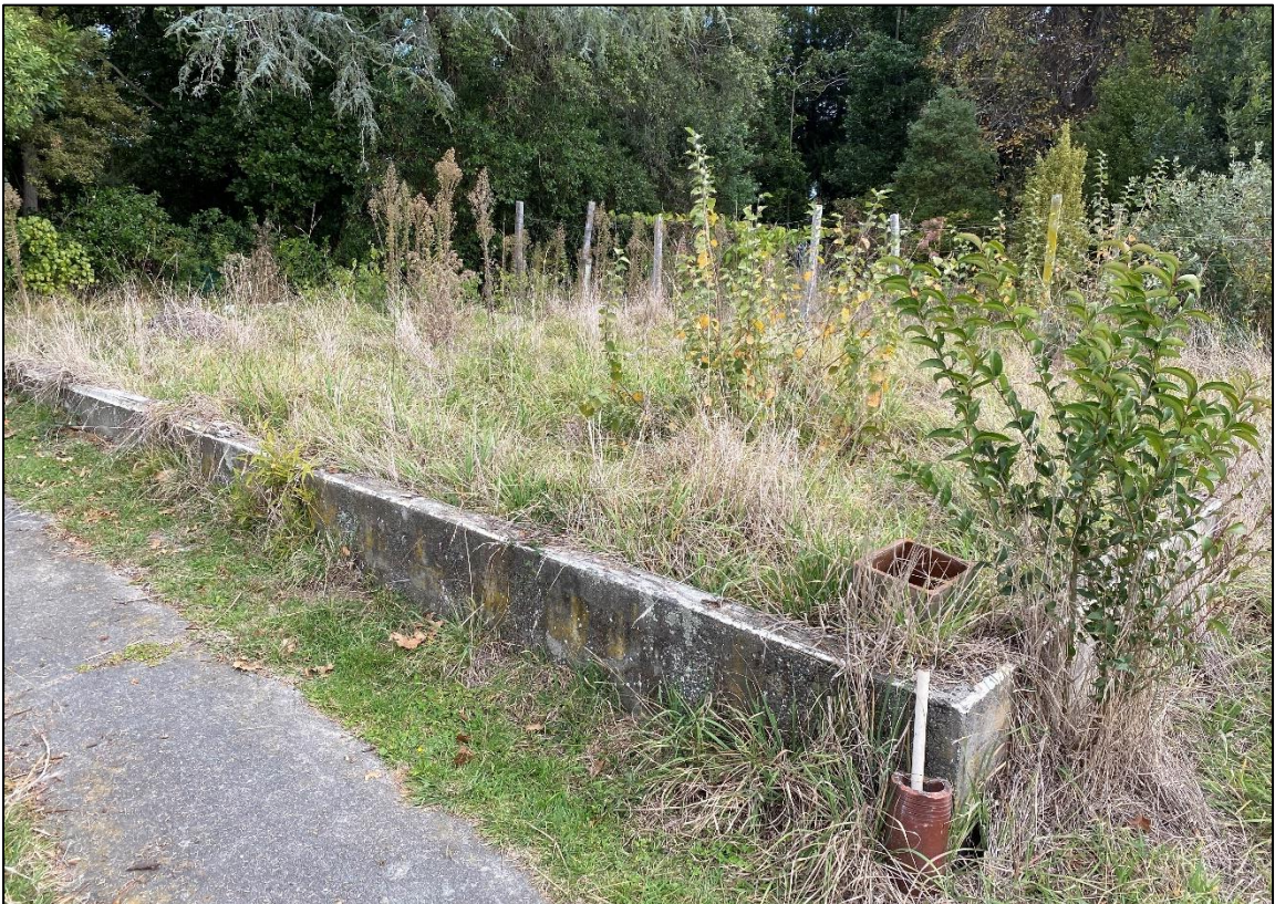
Photograph Appendix B.10: Concrete foundation of the former glasshouse at 76 Chesterhope Road.
