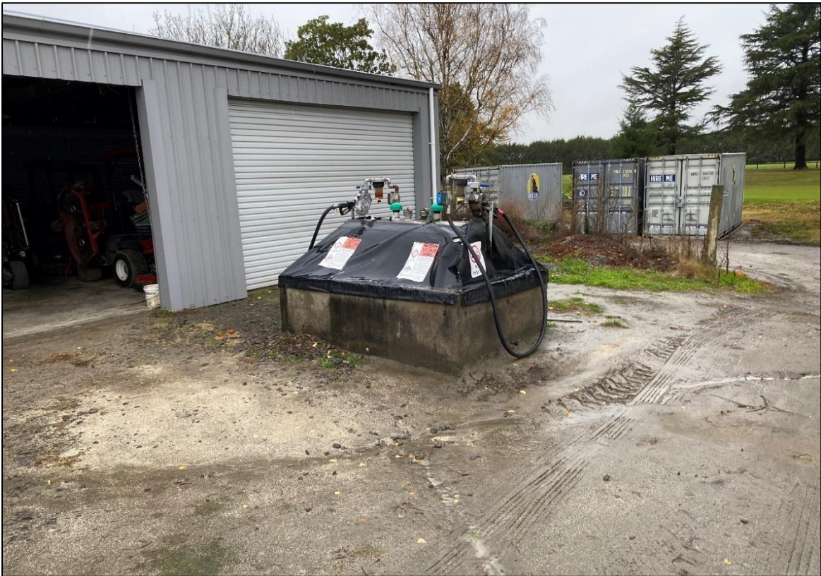
Photograph Appendix B.22: AST by maintenance sheds at golf club ( offsite ), looking south towards the site.
