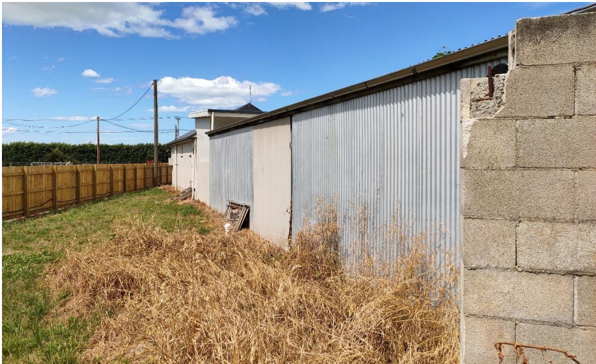
Photograph Appendix B.24: Site 7a – western side of Pakowhai Memorial Hall, facing north-east.
