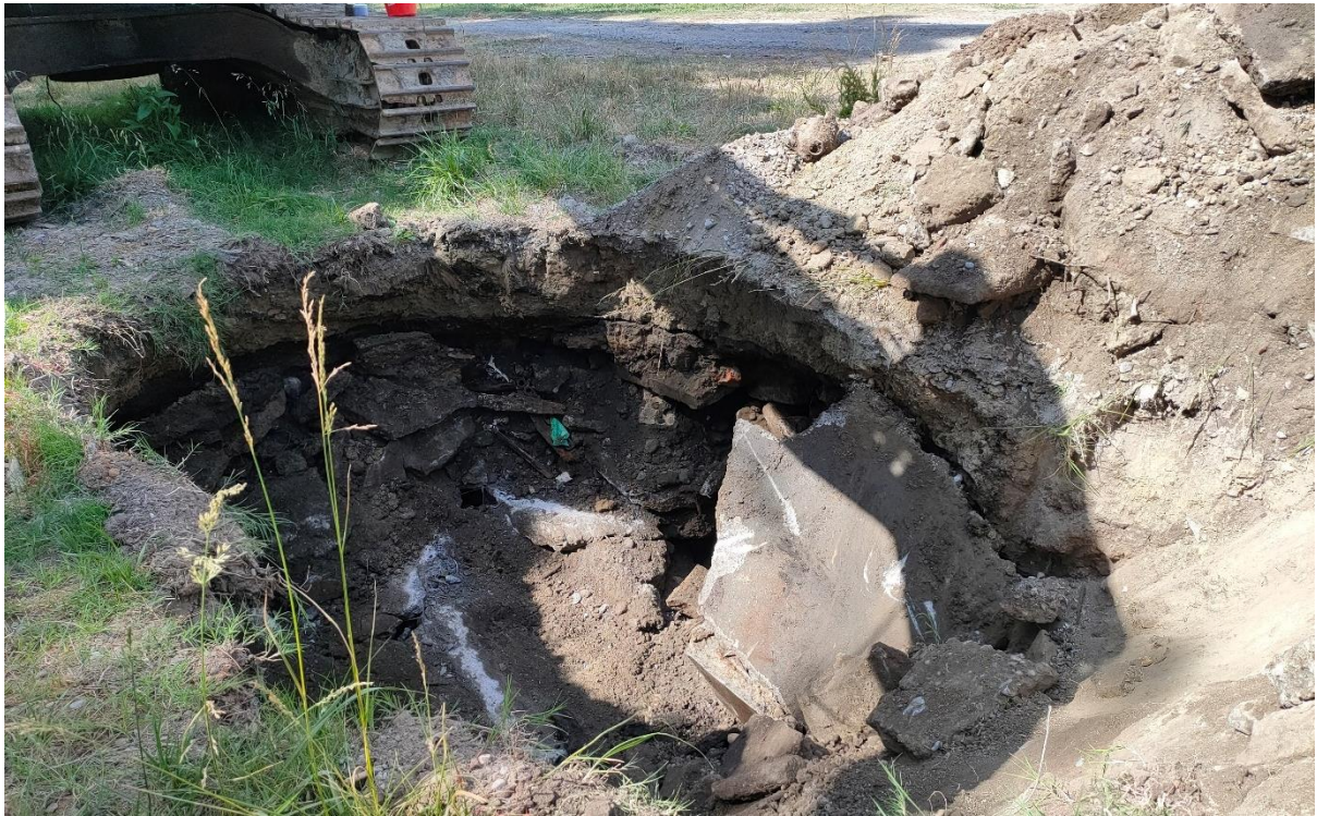
Photograph Appendix B.6: Site 2 – large concrete slabs in S2_TP4.
