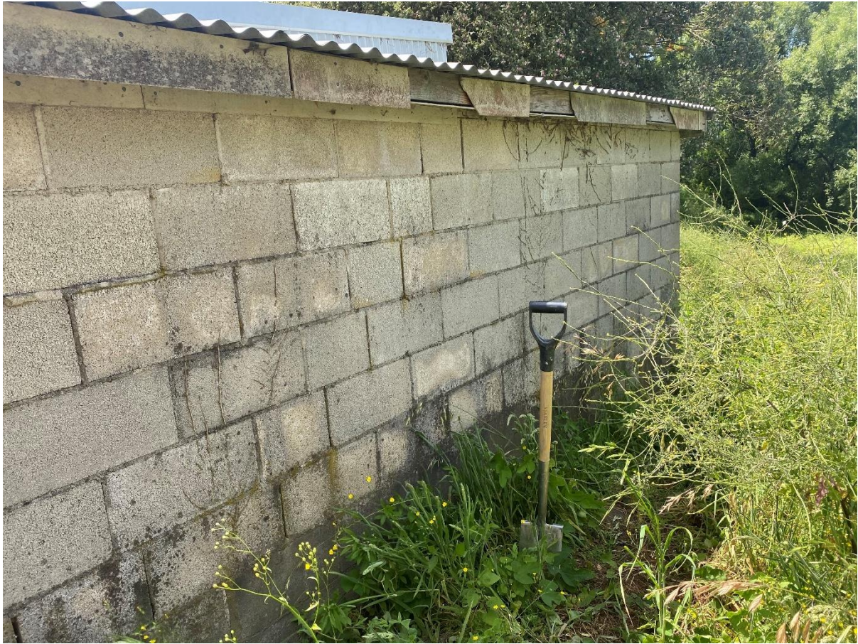
Photograph Appendix B.23: Site 7a – rear of Pakowhai Memorial Hall with damaged ACM fibre board cladding.
