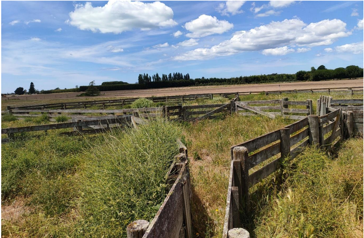
Photograph Appendix B.17: Site 4c and Site 7b – disused spray race/stockyard adjacent to woolshed, overgrown with grass and weeds.
