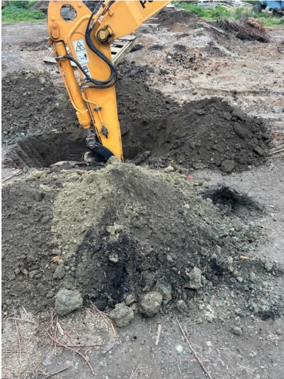
Photograph Appendix B.3: Location TP05 in Site 6 showing the encountered fill material.
