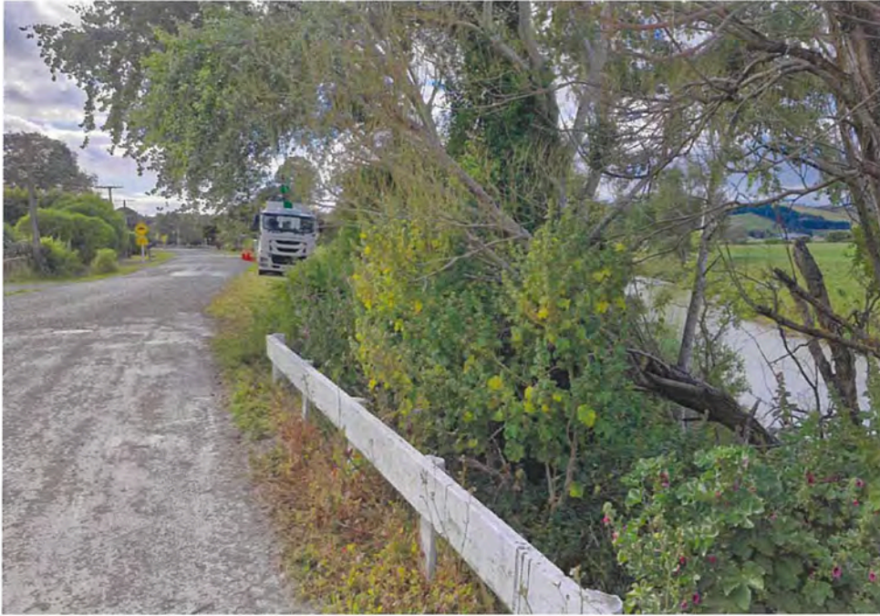
Photograph 7: Section 3 between Properties G and H - The photograph is taken from the northern side of the river, looking southeast (downstream) along the riverbank (site), with Keppel Street on the left of the photograph.
