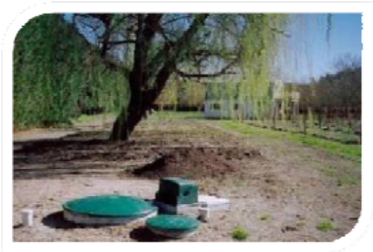
Parts of a secondary on-site wastewater treatment system that can be seen above ground.
