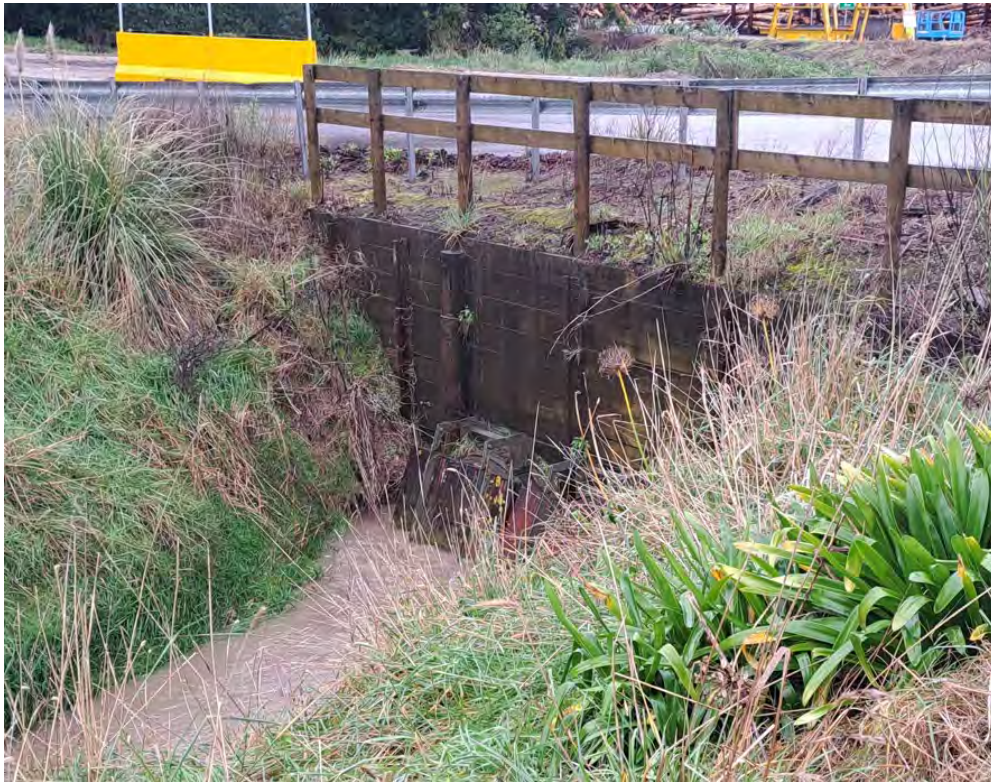
Photograph 9: Flap gate on the downstream side of the lower Pan Pac culvert.
