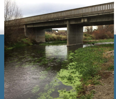
Above: Mangaonuku Stream at Tikokino Road. Below: Mangatahi Stream at The Brow Road.
