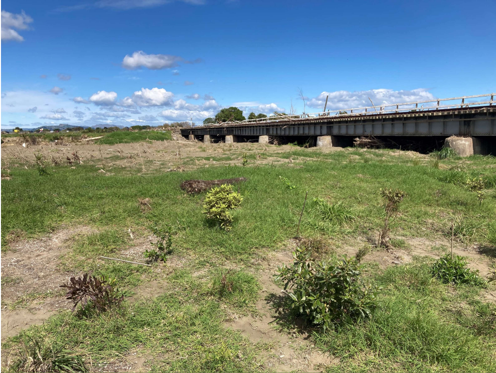
Downstream – Limited Capacity Note concrete piers are 3m tall less than 1m visible (photo 22/3/23)
